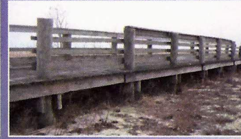
10 Boardwalk needs new railings & floorboards; supporting structure is in good condition
