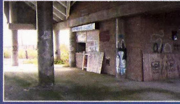
7 The Pavilion's facade has deteriorated, but its frame is structurally sound
