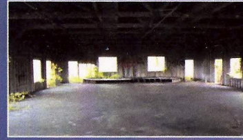
9 Structure needs further evaluation to determine if it can be salvaged for reuse
